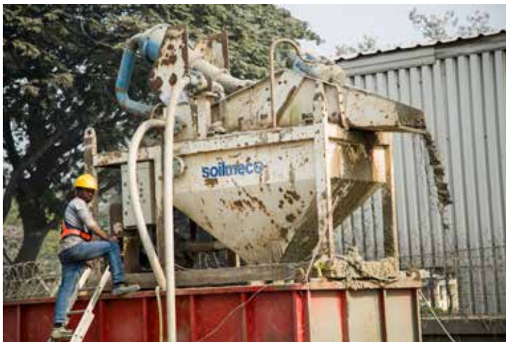
Desanding Unit at BAT, Kushtia.
